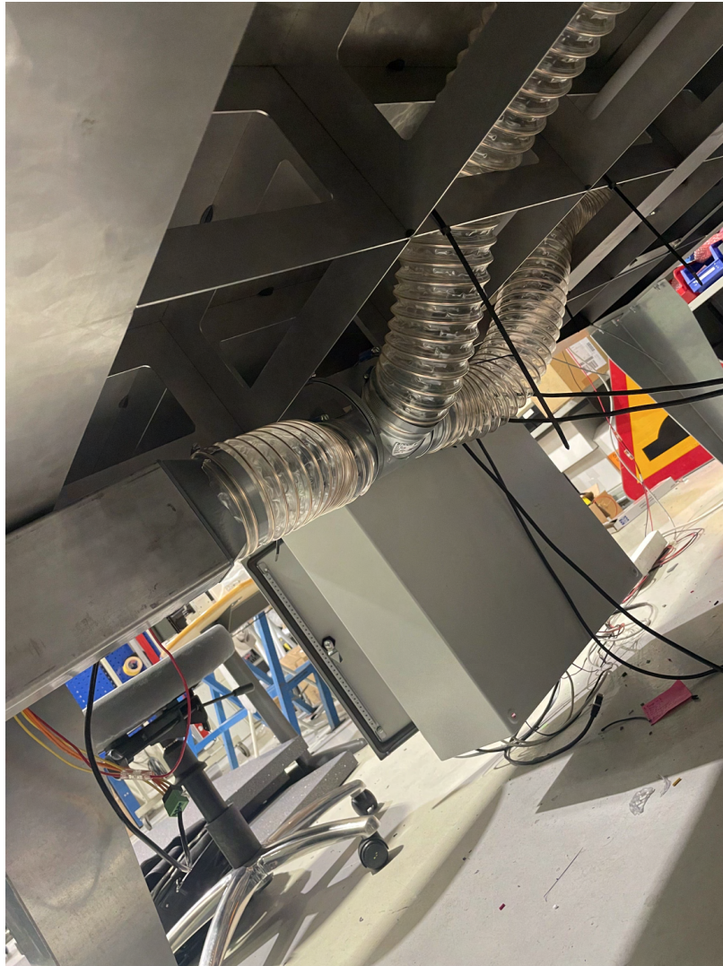
Figure 5.17: The T-connection of the ventilation system. The left pipe after the T-cross leads into the arm that the wire is mounted on. The right pipe leads to the box below the table.
